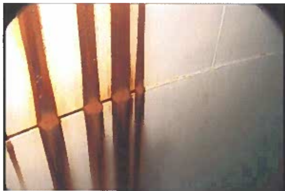
9:38 Corrosion cells on lower shell rings
