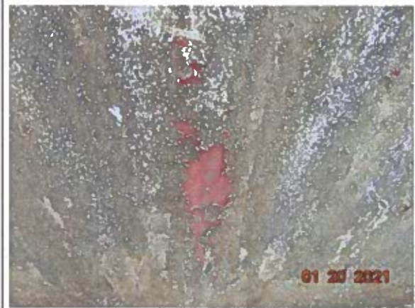
#8 Delamination on lower shell rings
