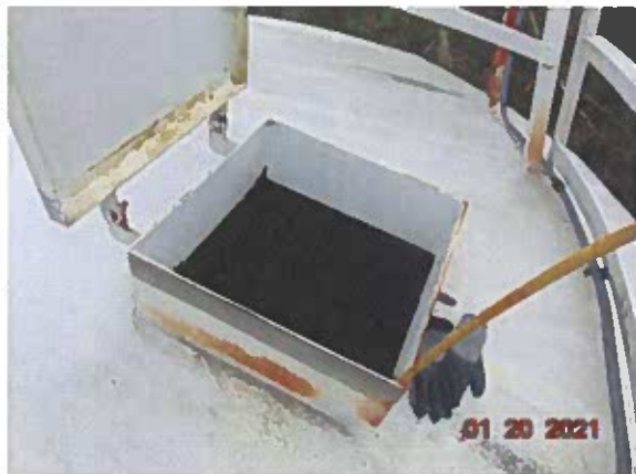
#20 Roof access hatch
