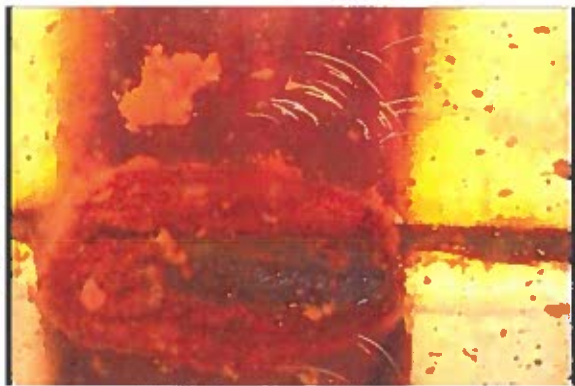
11:06 Exposed weld seam
