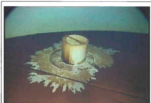
14:57 Inlet/outlet pipe with sediment ring
