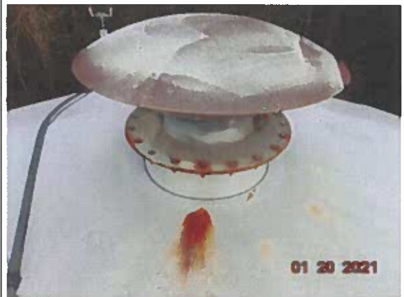
#17 Roof vent overview and corrosive staining
