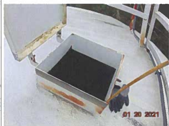
#20 Roof access hatch
