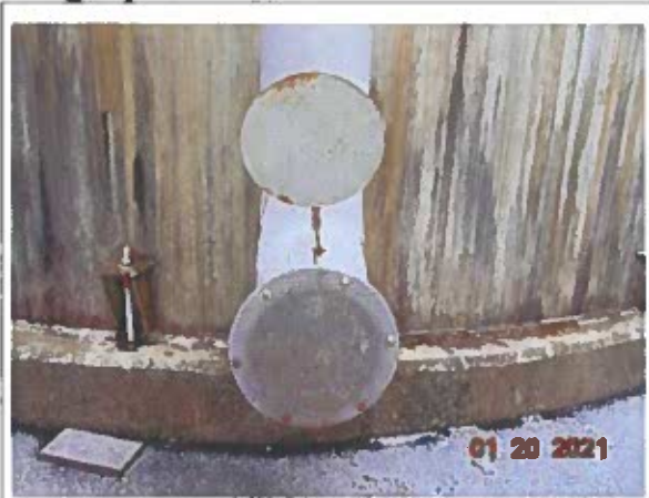
#4 Overflow with flapper valve and intact screen
