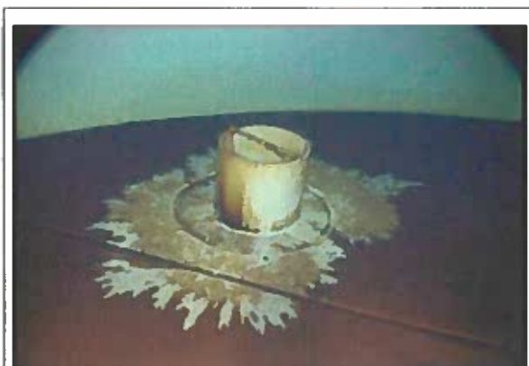
14:57 Inlet/outlet pipe with sediment ring
