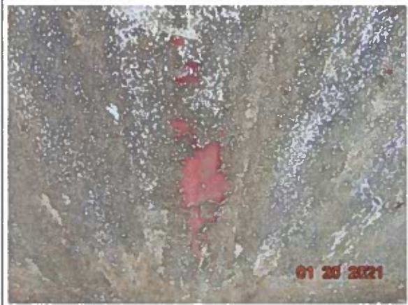
#8 Delamination on lower shell rings
