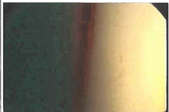
5:29 Staining on upper shell rings
