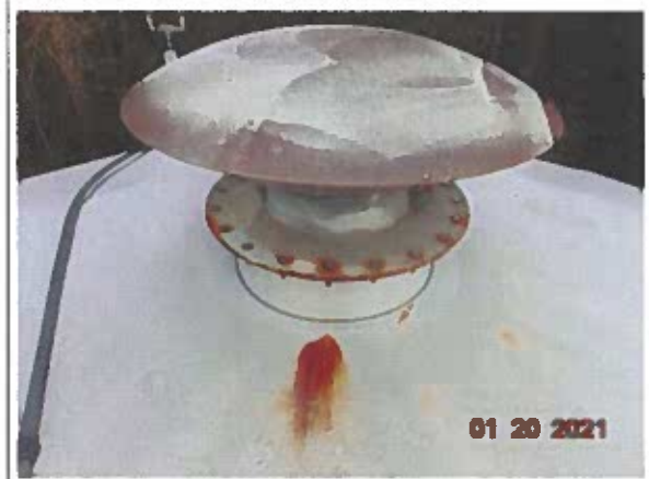
#17 Roof vent overview and corrosive staining
