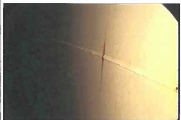
4:49 Corrosive staining from weld seam
