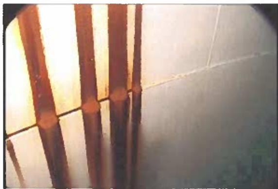
9:38 Corrosion cells on lower shell rings
